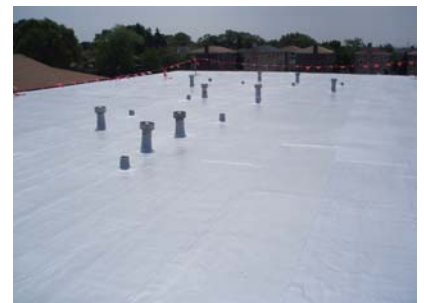
A completed roof is fully restored with a bright reflective surface that shields the existing roof from further UV damage. #3000 is completely waterproof and will withstand ponding water.
