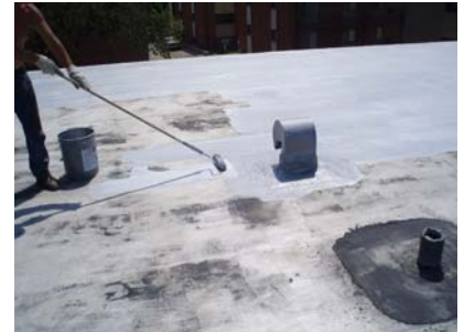
The existing APP modified bitumen roof has been power-washed with Lucas #115 Detergent Roof Primer. #3000 is applied by roller.
