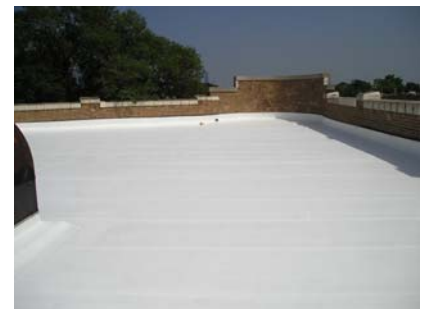
After a coating of Lucas #1000TC the same roof is sealed and protected with a cool white finish that will reflect heat away from the roof and prolong the roof's service life.
