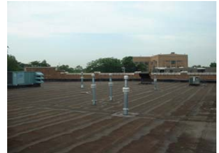
The existing un-coated modified bitumen roof has aged prematurely and appears brown from the oils that have 'cooked out' of the membrane.
